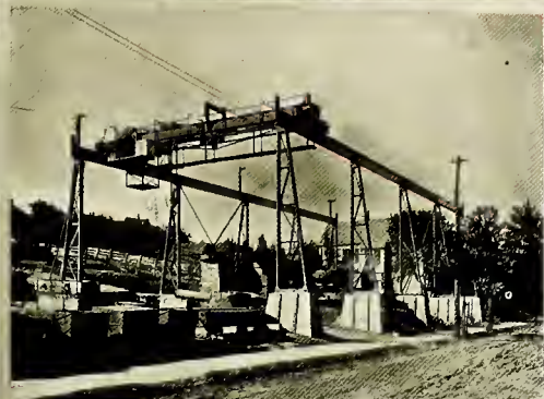
NEW ELECTRIC TRAVELING CRANE
